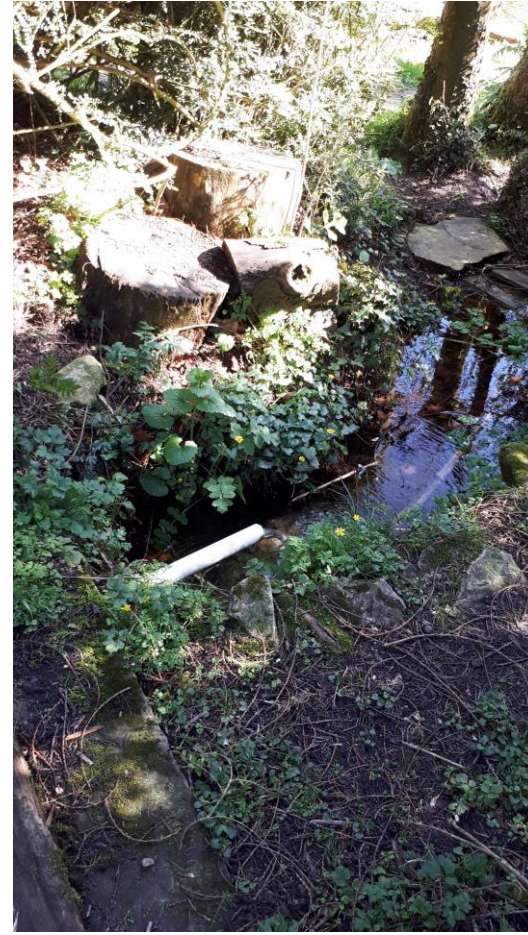
33_looking SE US extent of 31 where it is culverted under the road_180418
