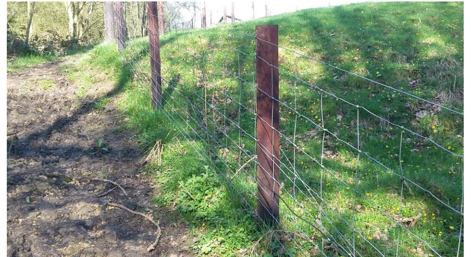
G36_seepage on banks of River Churn trib facing W
