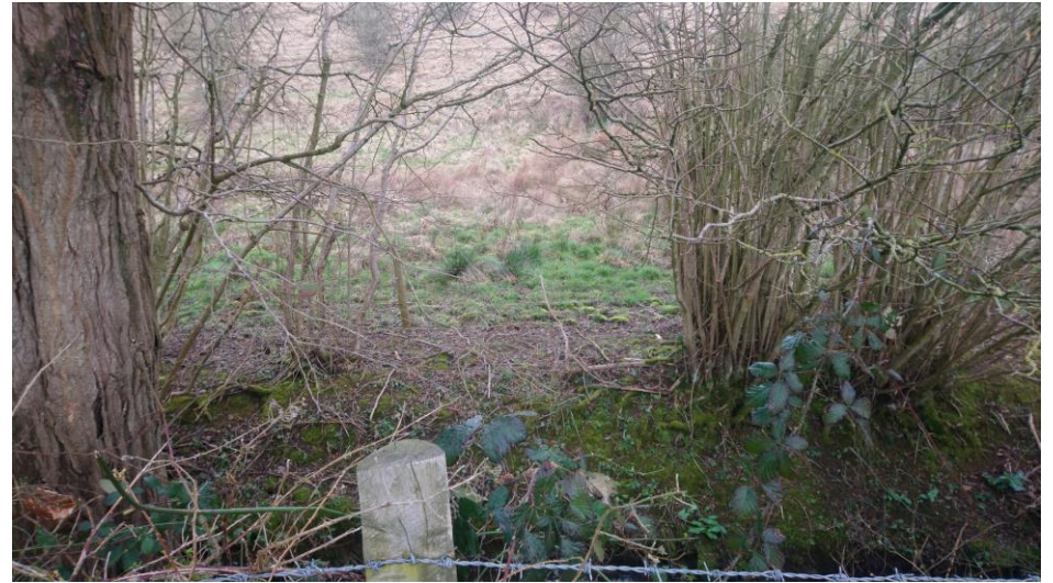
G137 _ possible seepage on L bank at Coldwell Bottom
