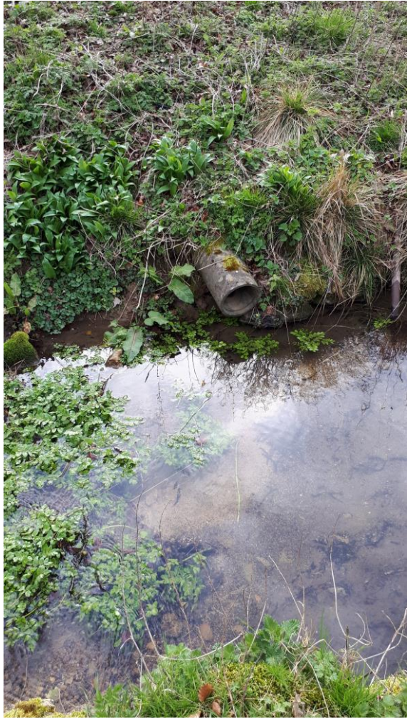
92_looking N US of 91_outfall likely from road drainage
