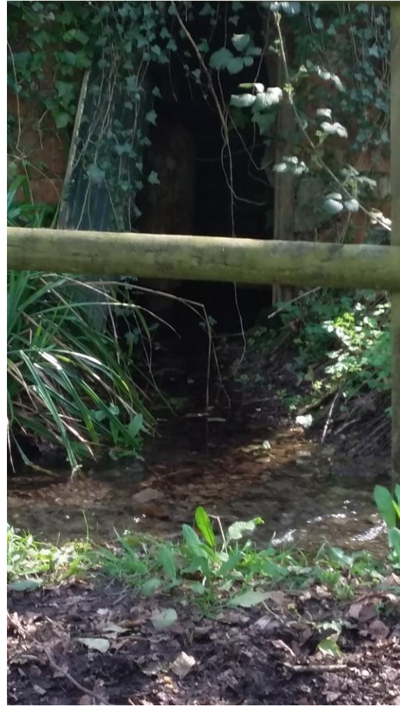
G47_spring fed flow and pump house facing E
