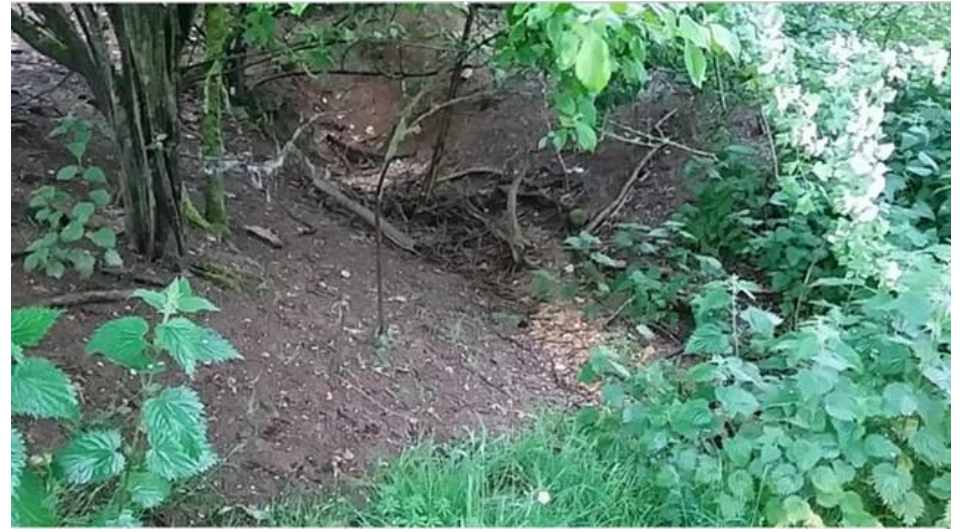
G77_watercourse seeps to ground marked as culvert but overgrown so not proved facing N W
